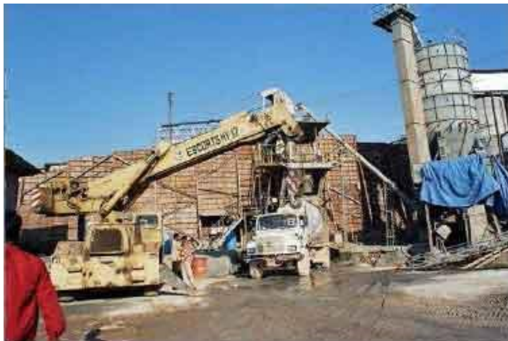
Fig. 89: Concrete-mixer on standby of loading. Machine preparation of the concrete. Source: CREMIN Emilie, March 2005.
