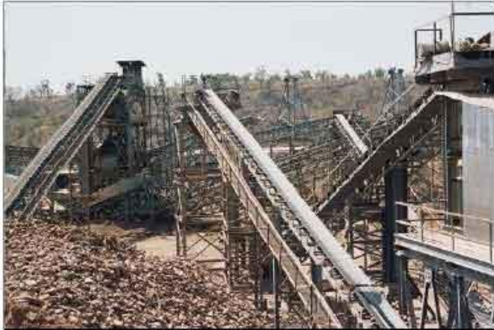
Fig. 88: Temporary installation on northern bank of Narmada close to the village of Siddhavarakuta. Machine preparation of the concrete (crushing) for the construction of the power station. Source: CREMIN Emilie, March 2005.
