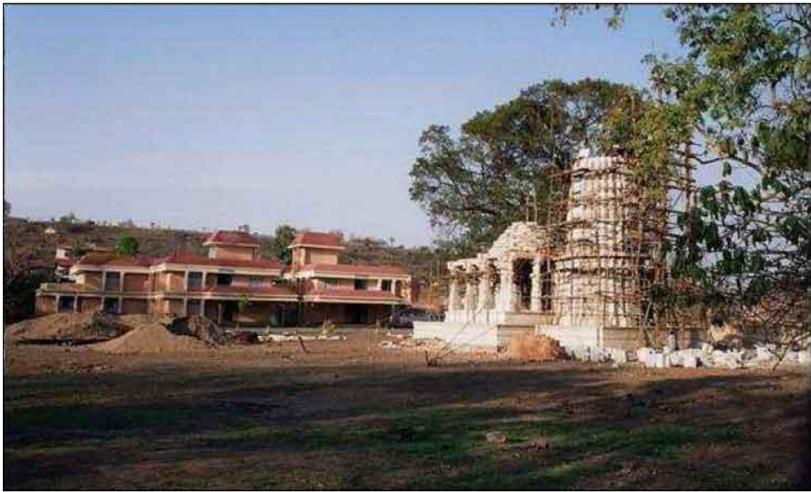
Fig. 106: Temple of Ashram Gajanan Maharaj in the course of construction. Source: CREMIN Emilie, March 2005.
