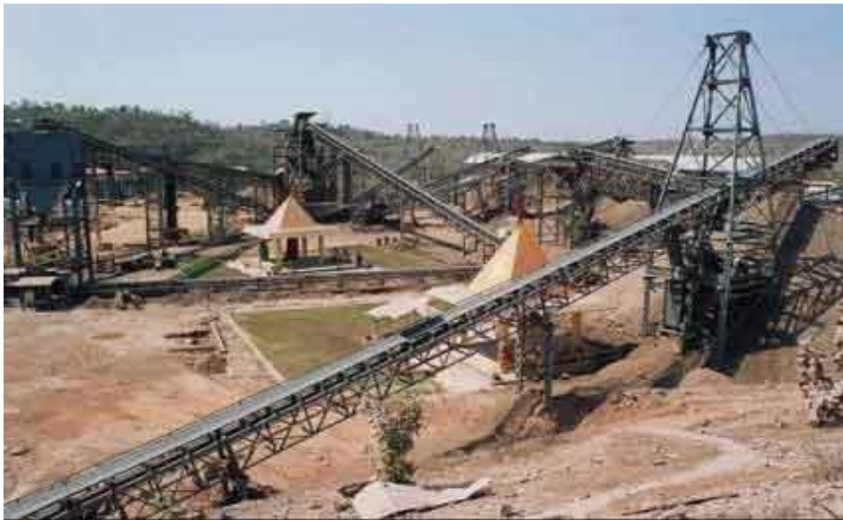
Fig. 87: Building site of the dam. Temporary installation on northern bank of Narmada close to the village of Siddhavarakuta. Machine preparation of the concrete (crushing) for the construction of the power station. In the center, two temples containing the sculptures of Hindu divinities, vestiges of the old temples which were located in this site before the beginning of work. Source: CREMIN Emilie, March 2005.
